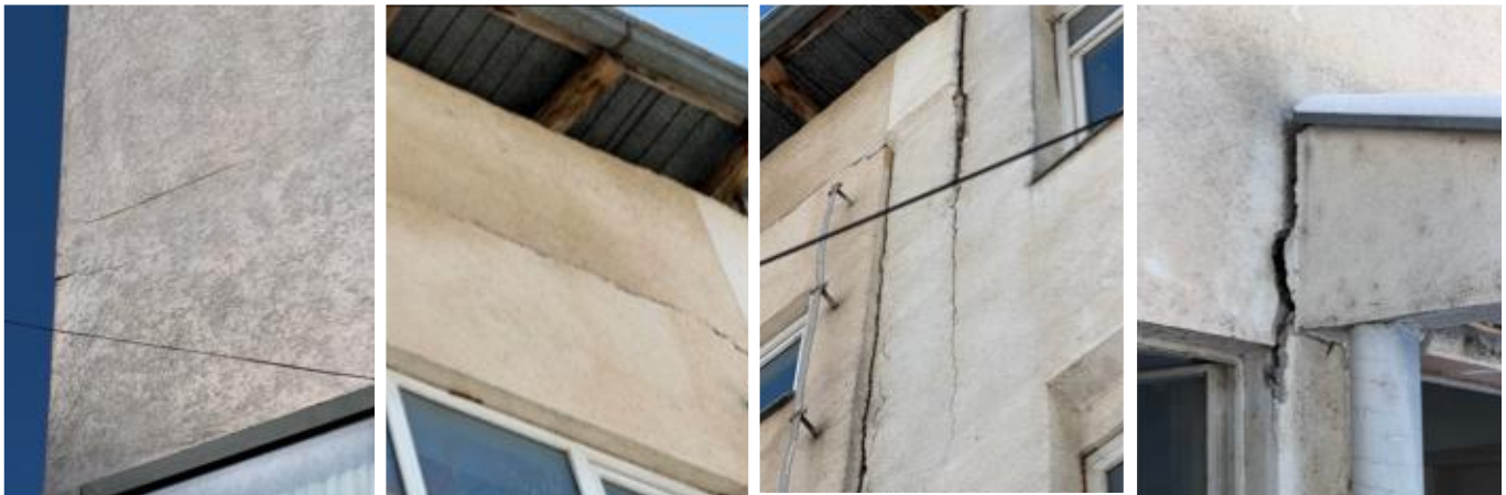
Figure 2. Representative facade images illustrating variations in crack thickness and local shadowing effects within the dataset.
